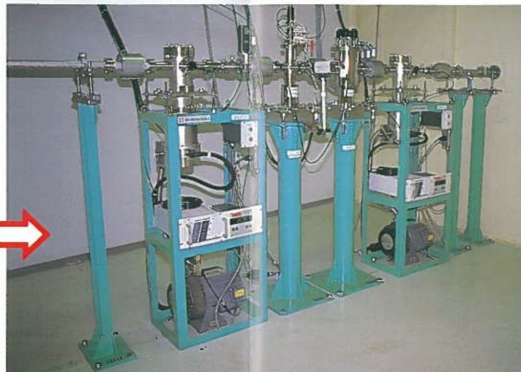
▲A beamline with evacuation units installed at about 5 meter intervals.
